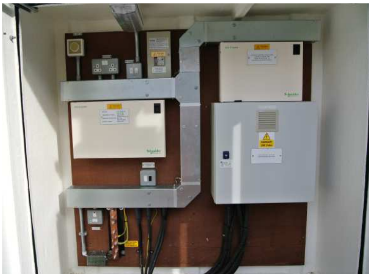
Typical feeder pillar installation.
